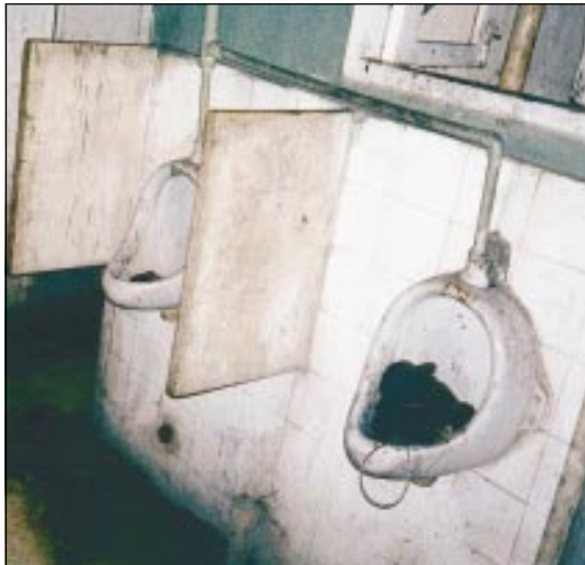
Blocked toilets at the Indira Gandhi Children's Hospital
