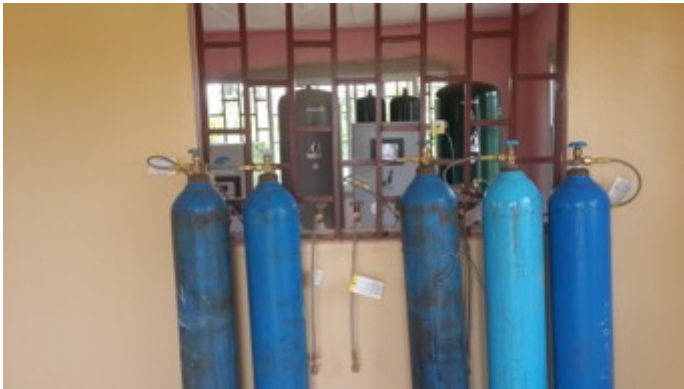
Because of the unreliability of electrically powered oxygen supply systems (oxygen concentrators), during the Ebola outbreak, MCAI provided an oxygen generator system based at Phebe Hospital that produces large cylinders full of medical grade oxygen for 4 nearby hospitals, including CB Dunbar Hospital
