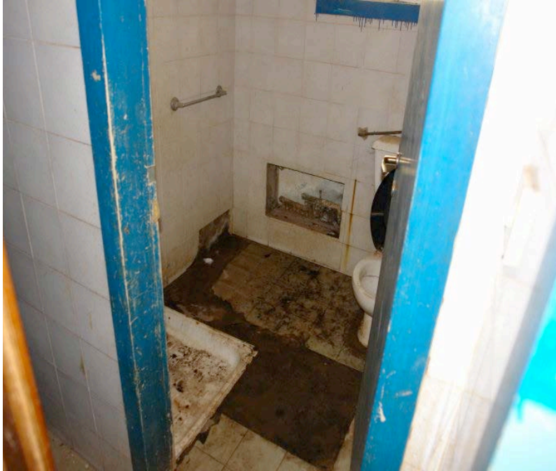
A very dirty toilet; a common finding in public sector hospitals of poorly resourced countries
