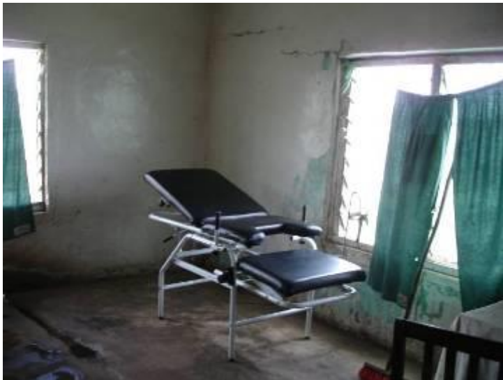
Labour ward in a health facility. No resuscitation equipment for the newborn infant
