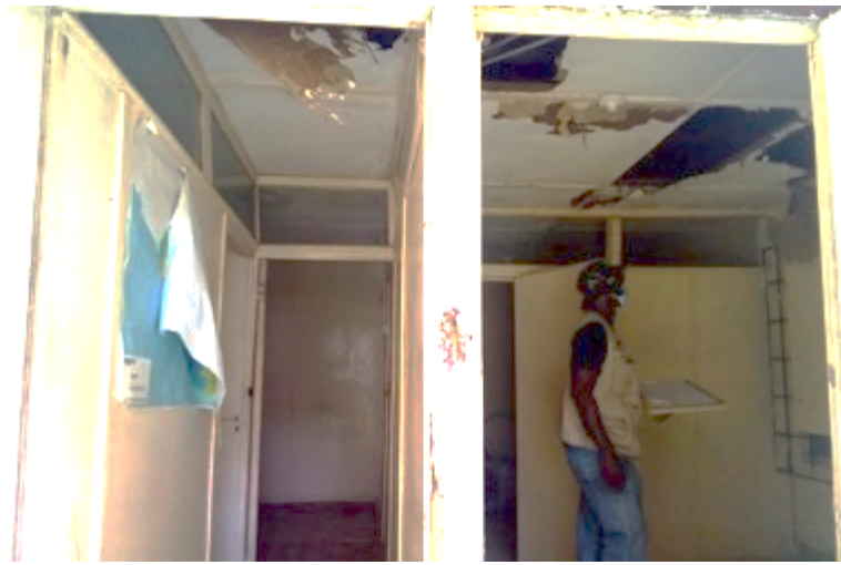
ABOVE: Before renovation: asbestos in the roof over the children's ward
